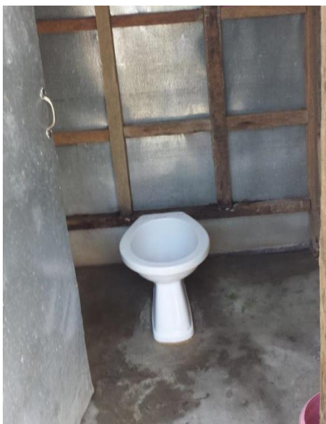
Figure 7-1 Typical toilet pedestal in use in Abucay Bunkhouse (Photo: F. Zakaria)
