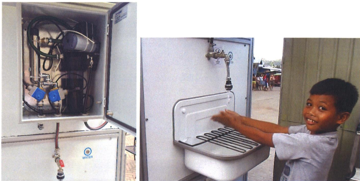
Figure 3-23 Mini unit for service water treatment (left) and a child using the hand washing facility (right)(Photos: F. Zakaria)
