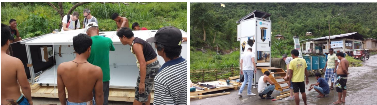
Figure 3-37 Assembling the toilet on-site with the help of local community (Photos: F. Zakaria)
