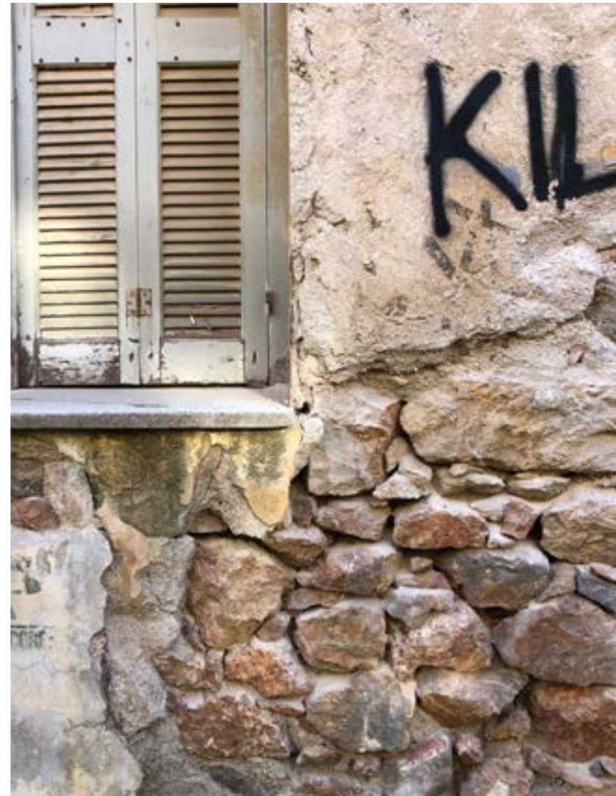
Image 3.25b. Author (2021). Current condition of north facade [Photograph].
