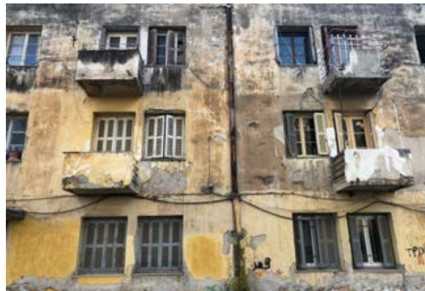
Image 3.6. Author (2021). Current condition of the north facade of the last building of “Prosfygika” on Trixonidos Street.
