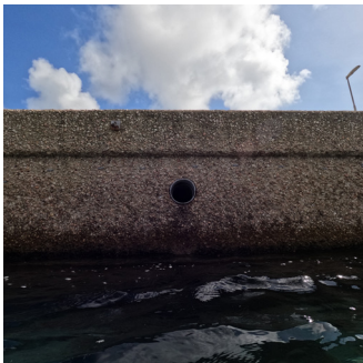
zone 2 | drainage system outlet
