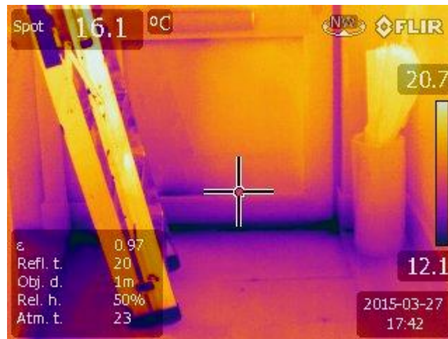
Fig. 76: Front door corridor infrared image
