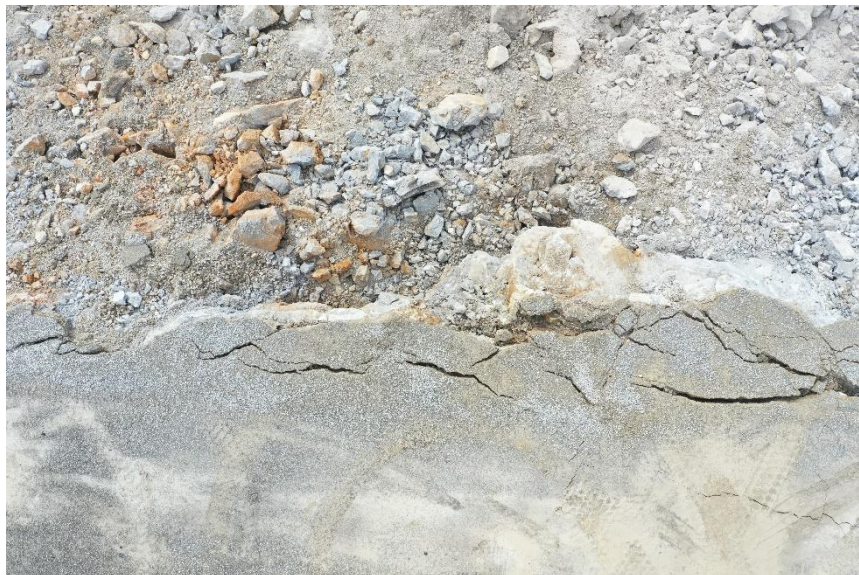
Figure 39 Example Image showing cracks post blasting in the crest region
