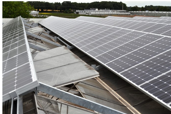
Figure 3.6: c-Si modules installed on assembly rack on top of greenhouse roof [136]
