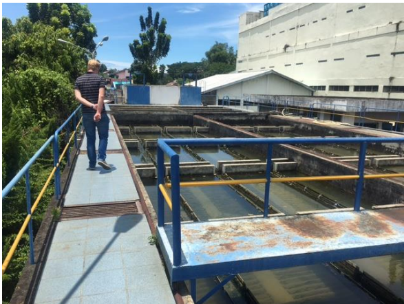
Figure 31: Part of the treatment plant Paal II
