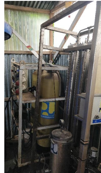
Figure 37: Leftovers of RO installation number 3
