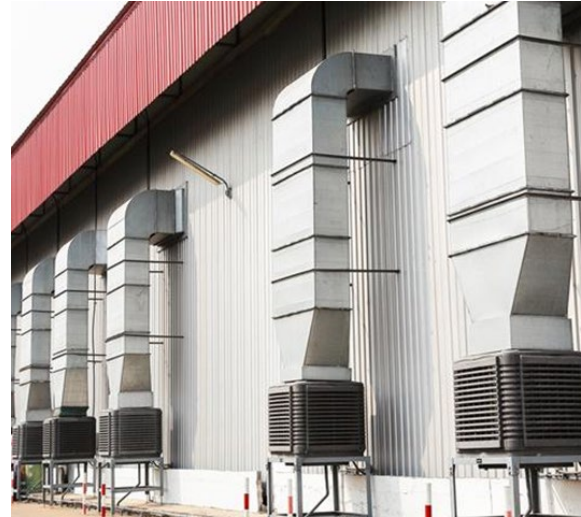
Figure 5.6. Modern evaporative cooling units on the facade of a building.
