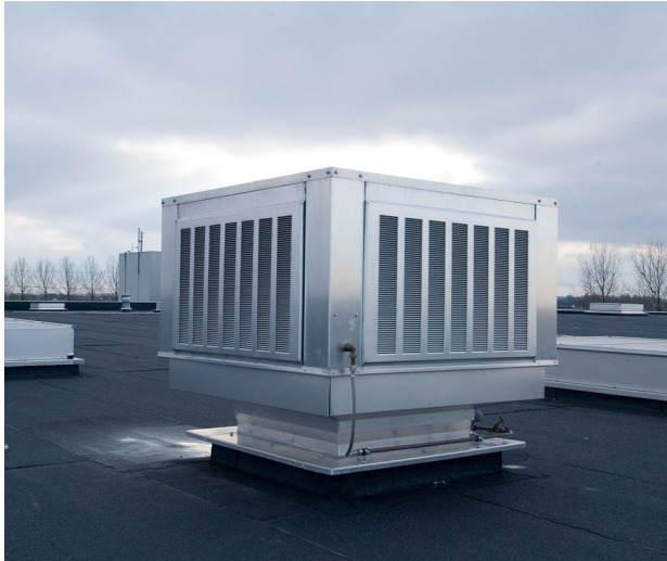
Figure 5.5. A modern evaporative cooling unit on the roof of a building.
