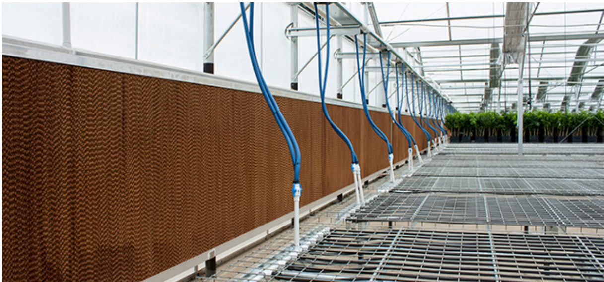
Figure 5.7. Evaporative cooling pads applied to the side of a green house.
