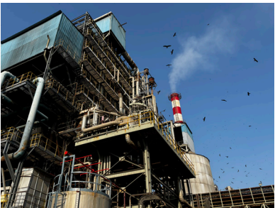
Incinerators and waste compressors
