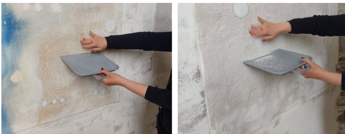
Fig. 9. Left: Panel A1: No loss of cohesion of the plaster; Right: Panel A2 significant sanding of the plaster; Situation 48 months (t48) after the application.
