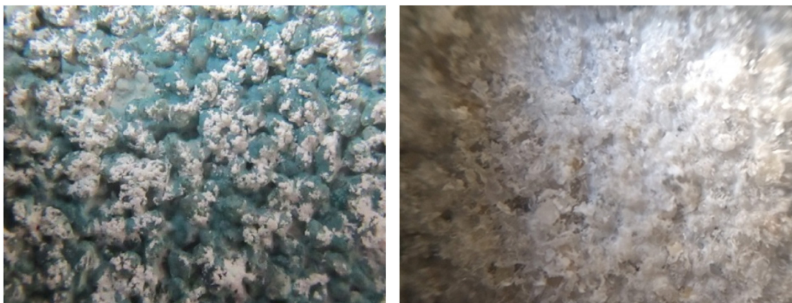
Fig. 8. Left: Dendritic salt efflorescence on panel A1, 3 months after the application; Right: salt crust on the surface of panel A2, 6 months after the application (right).
