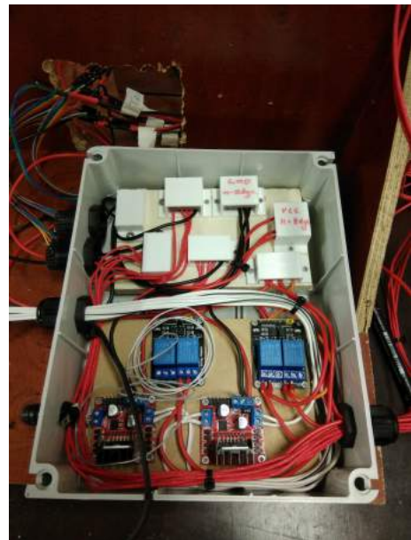
(b) The wiring of the power circuit housing.
