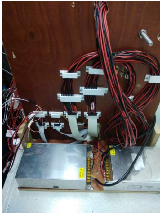
(a) The temperature sensor wiring behind the reactor.
