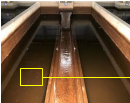
Figure 97a Full-scale RSF during ETSW 5 m/h up-flow
