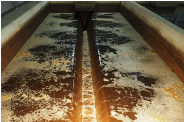
Figure 96 Full-scale RSF during collapse pulsing 40 m/h backwashing scour
