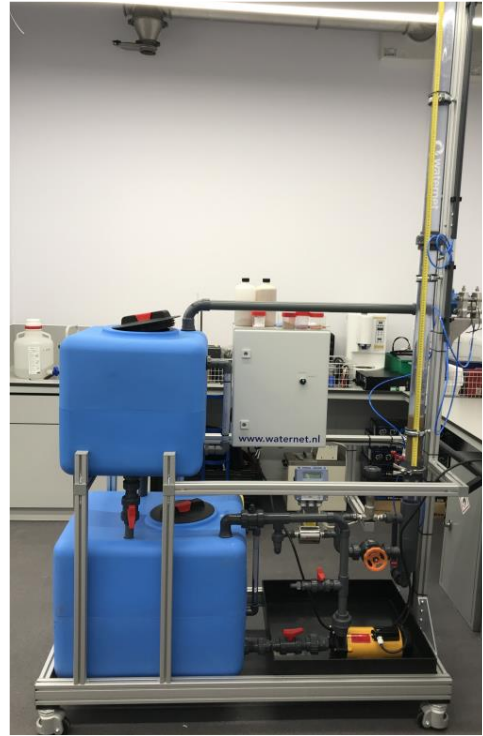
Figure 10 QMUL mobile expansion column in London
