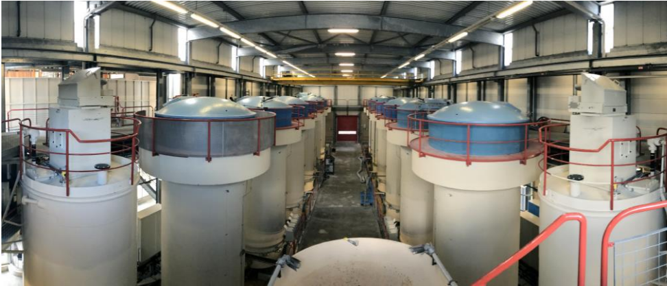
Figure 111 Full-scale pellet-softening reactors located at Waternet (Leiduin, The Netherlands) (van der Veen and Graveland, 1988).
