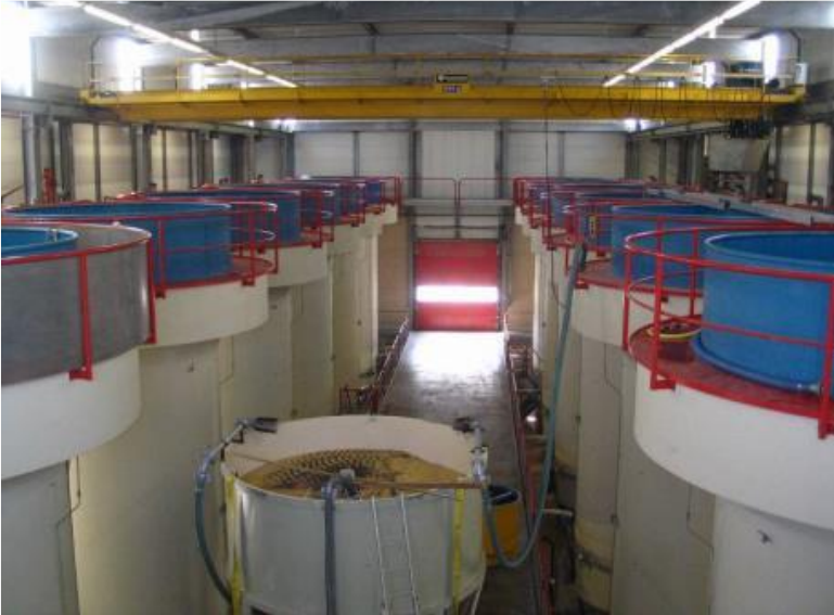
Figure 65 Full-scale pellet-softening reactors located at Waternet (Amsterdam, the Netherlands). The unit consists of 12 Amsterdam reactors with reactor diameter D = 3.0 m (van der Veen and Graveland, 1988).
