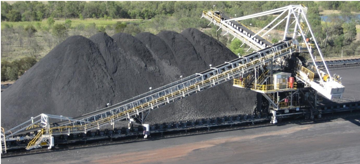
Figure 6.3: Stacker with a tripper car (Courtesy of ThyssenKrupp)
