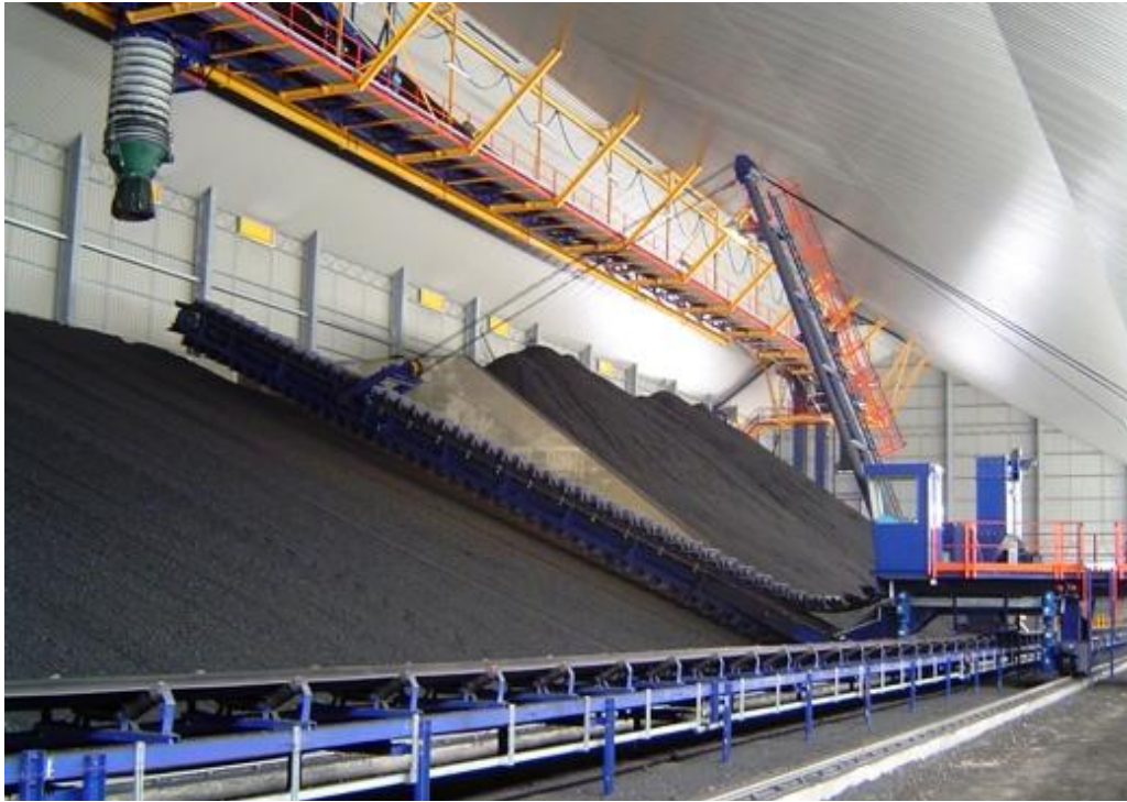
Figure 6.5: Stacking of coal using an overhead conveyor with telescopic loading chute and a side scraper reclaimer (Courtesy of Taim Weser)
