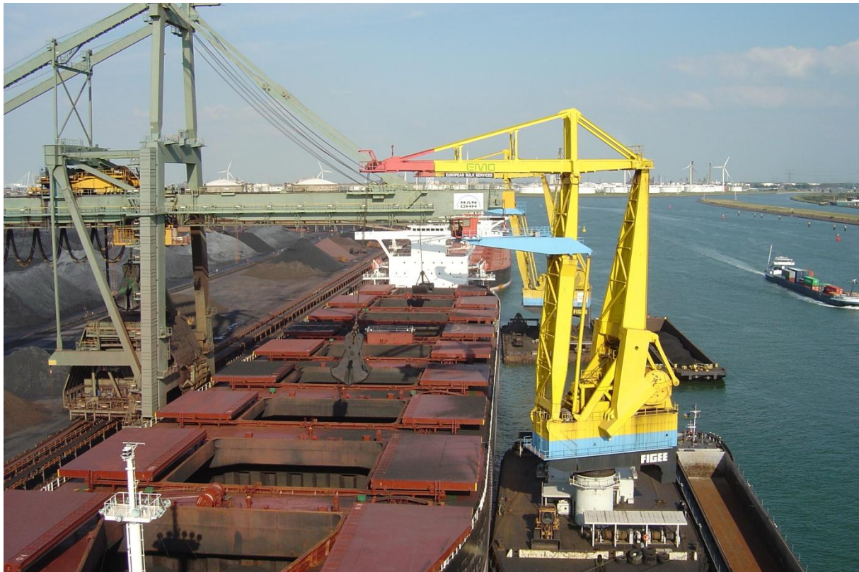
Figure 3.4: A rail-mounted grab crane and pontoon-mounted slewing grab cranes unload a bulk ship simultaneously (Courtesy of EMO BV)
