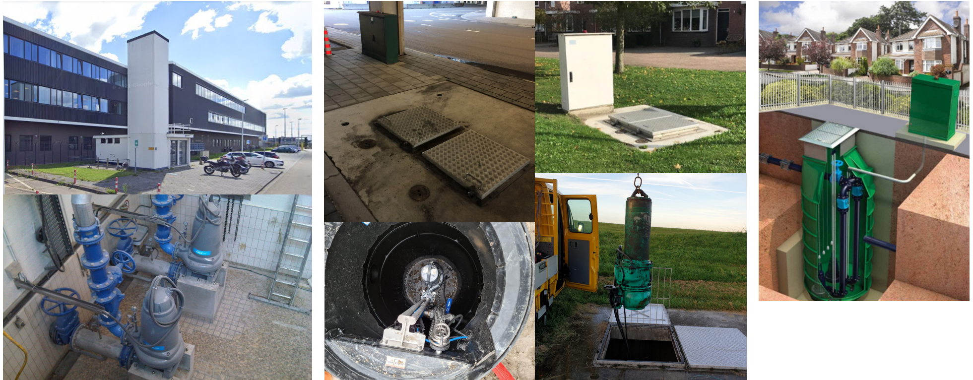
Figure 2: Wastewater pumping stations. From left to right: a main pumping station at Schiphol, examples of lower pumping stations and a schematic overview of the visible and invisible components of a pumping station. The lower images give a good indication of the size of the pumps.
