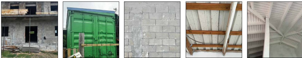
FIG. 4.7 Structure Suit: Ranks, and Options. Examples: (a) concrete structure; (b) metal structure; (c) concrete blocks wall; (d) wooden flat roof; (e) wooden gable roof.
