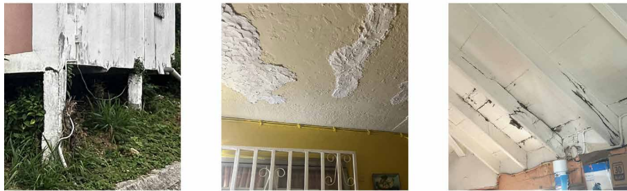
FIG. 3.8 Examples of damaged elements (A) damaged concrete piles; (B) patched concrete ceiling; (C) damaged wooden rafters.
