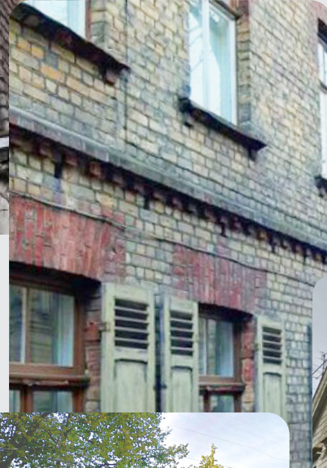
Excessive use of brick
