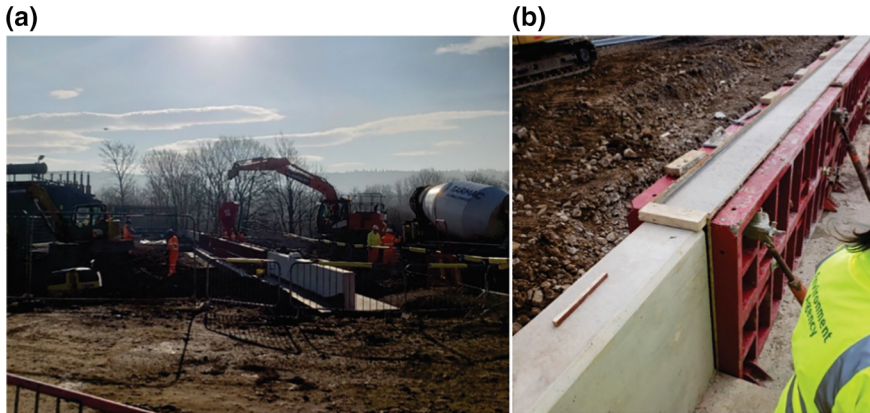
Fig. 13 a Placing the product via a concrete skip and b Finished product (in the formwork) [16]. Foto archive of Dr. Kanavaris
