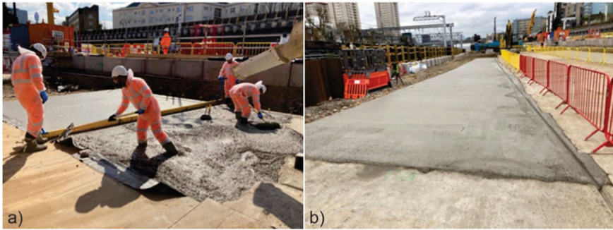
Fig. 9 a Depositing the product via the concrete truck's chute and b the finished product. Foto archive of Dr. Kanavaris
