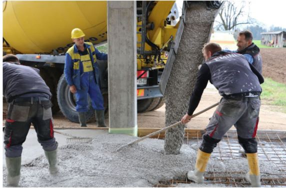
Fig. 6 Casting the concrete floor slab in Kranj (Slovenia) as a part of EConcrete project [11, 12]. Foto archive of Zevnik lab
