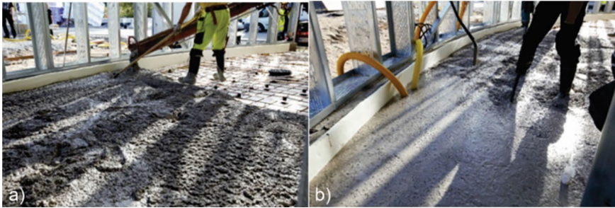
Fig. 7 a Casting the concrete and b vibrating the concrete to reduce air entrapment. Foto archive of Tero Luukkonen
