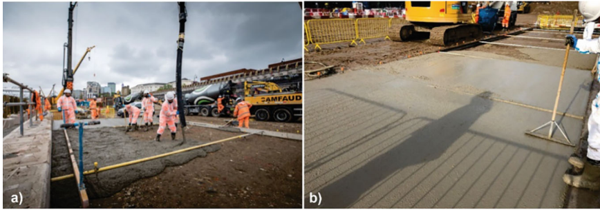
Fig. 8 a Placing the product using a pump, b finishing the surface. Foto archive of Dr. Kanavaris
