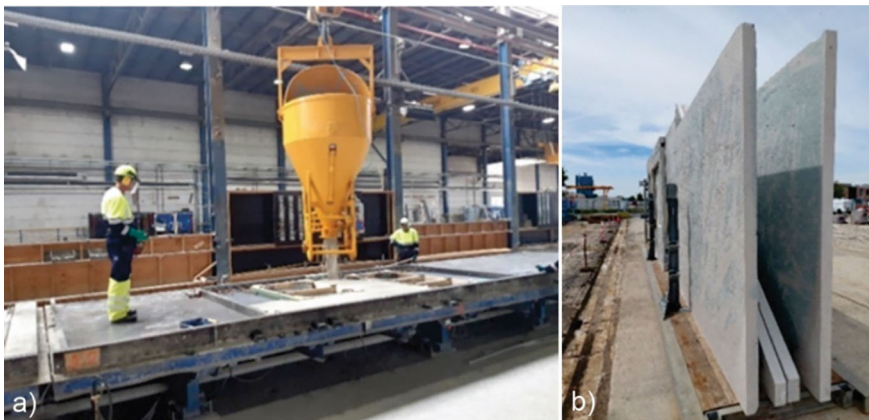
Fig. 2 a The pre-casting procedure and b the precast concrete walls. Foto archive of Arno Keulen
