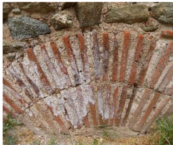
Fig. 31 Efflorescence near to the ground level
