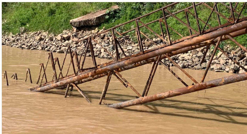
Figure 5.15: Close view of the collapsed bridge
