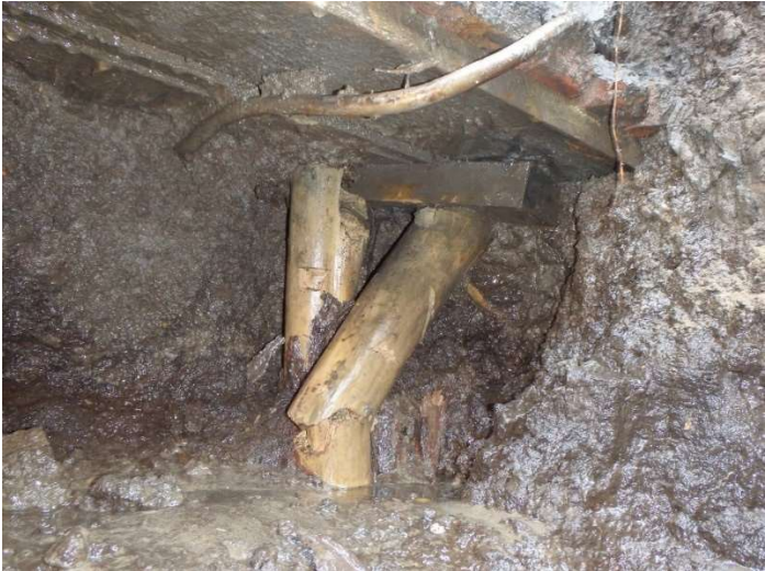
Figure 2 Broken wooden foundation piles (source: Fugro)
