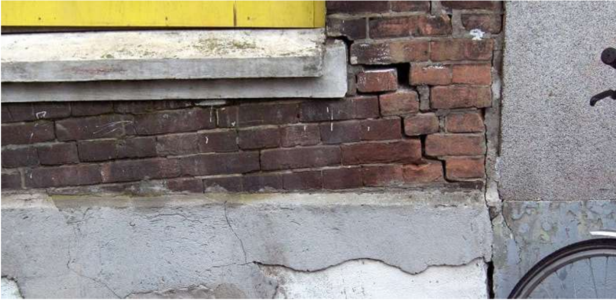
Figure 1 Cracks in the façade caused by settlement. (source: kcaf.nl)
