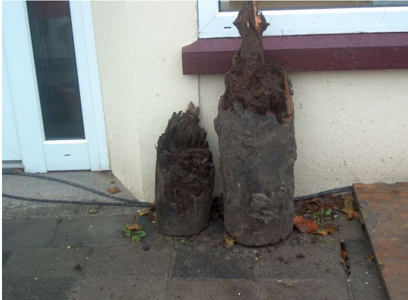
Figure 8 Fungus attack on wooden pile (source: Platform Fundering)
