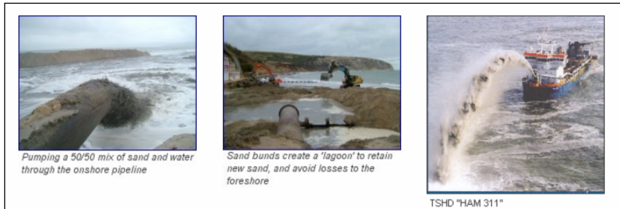
Figure 2. Examples of beach replenishment methods being used at Bournemouth (taken from Poole Bay and Swanage Beach Replenishment Website, 2006).
