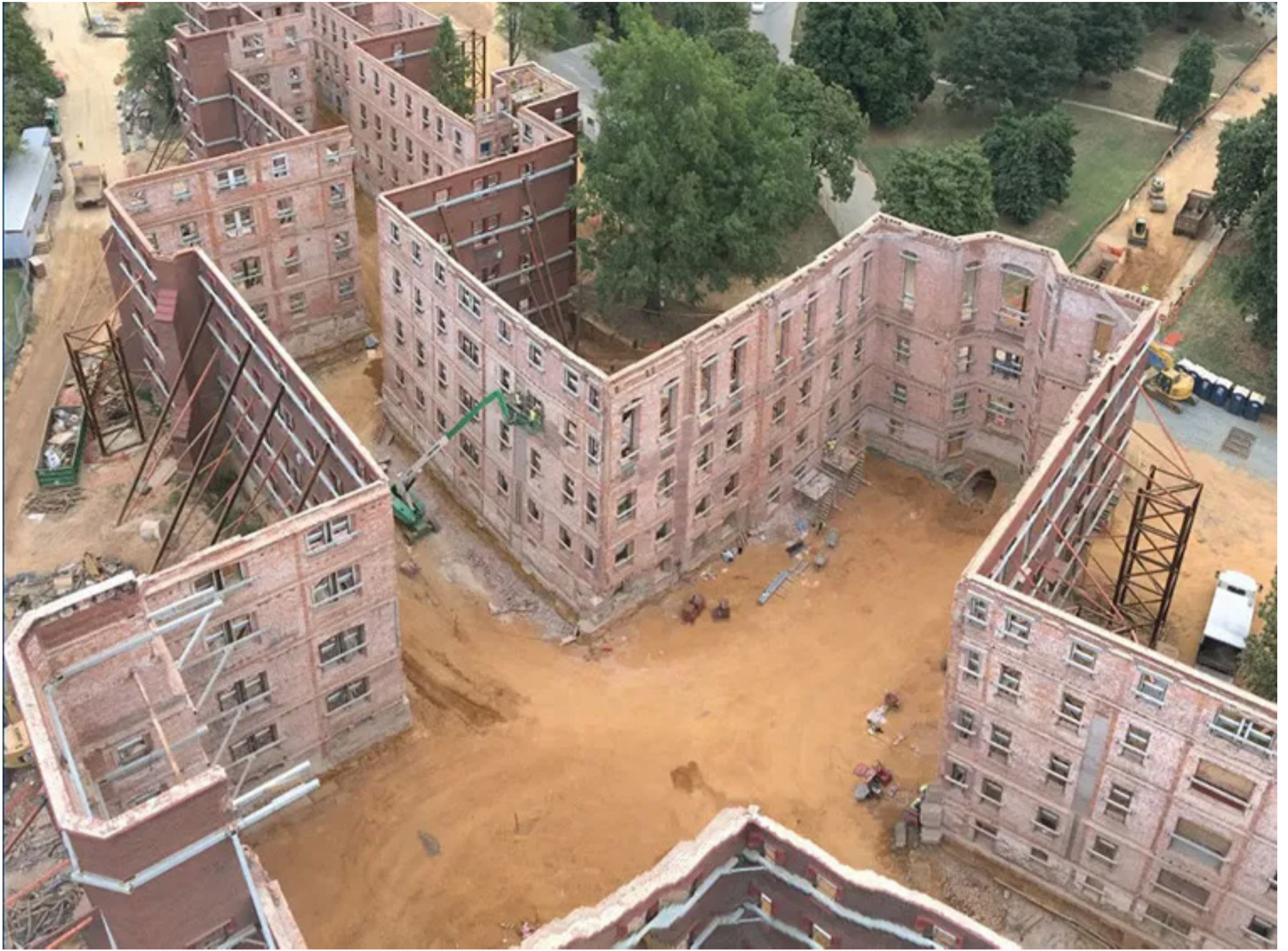
Façade ruin. St-Elizabeth's Hospital renovation, Washington DC
