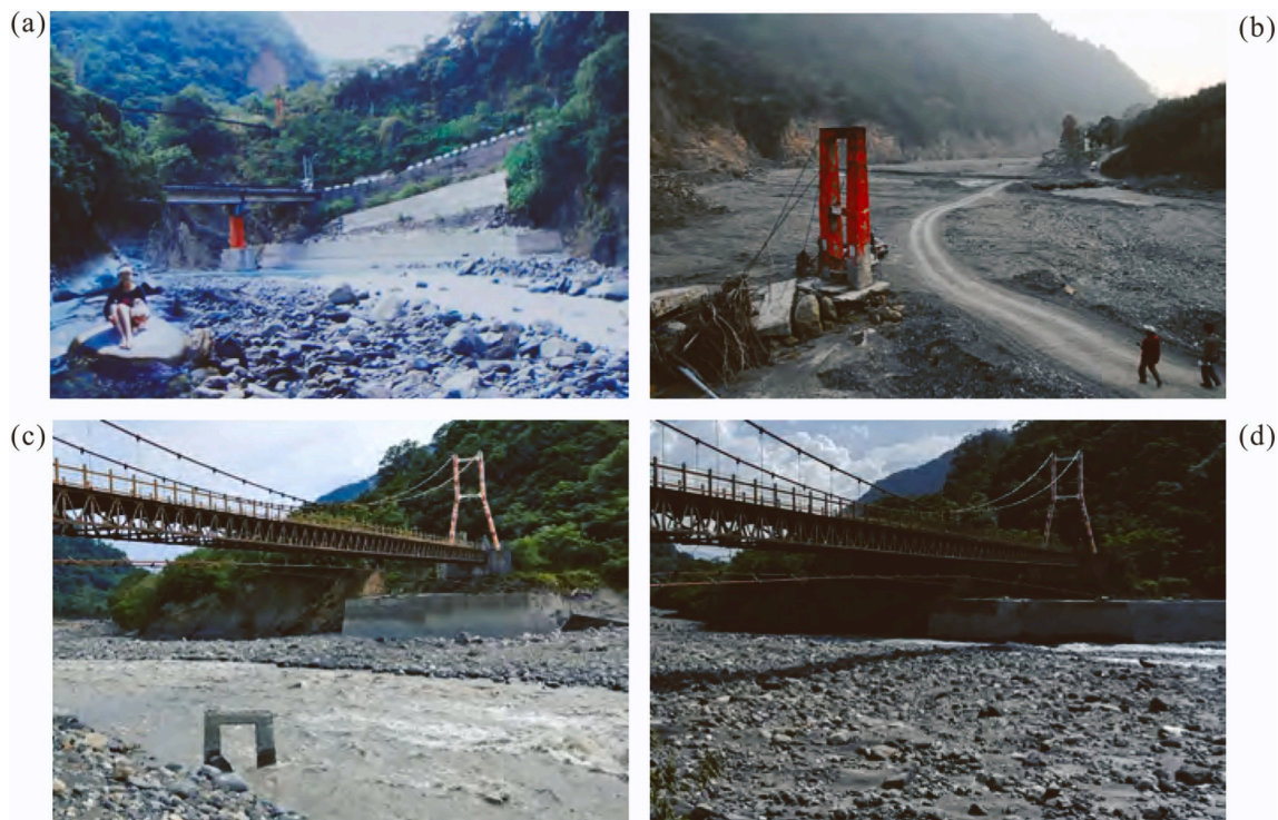
Fig. 1. Risk to infrastructure due to river bed elevation change, as illustrated by the Laonong River at the Aqiba bridge site: (a) before 2009 (roadside hot spring advertisement); (b) in February 2010, after the Morakot geomorphic flood; (c) in September 2019; (d) in August 2021 (see text for description).
