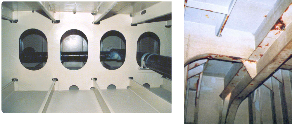
Figure 1 New ballast water tank & in "GOOD" condition after 15 years
