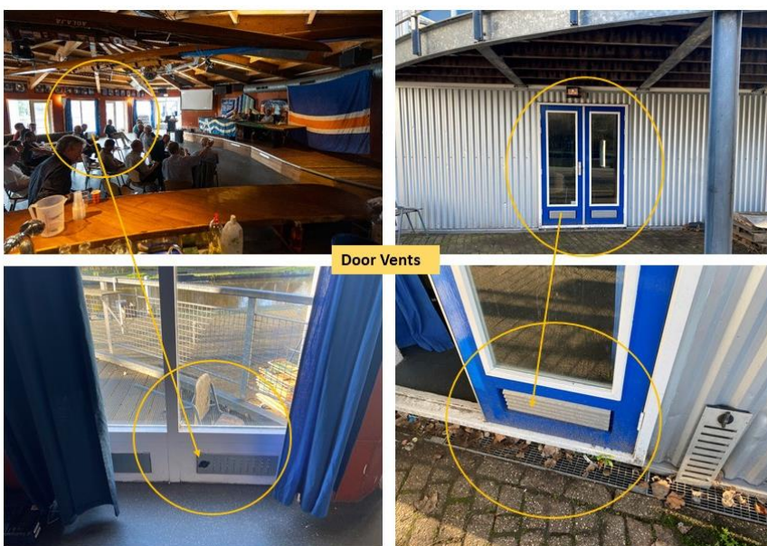
Figure 47 Natural ventilation through grills in doors
