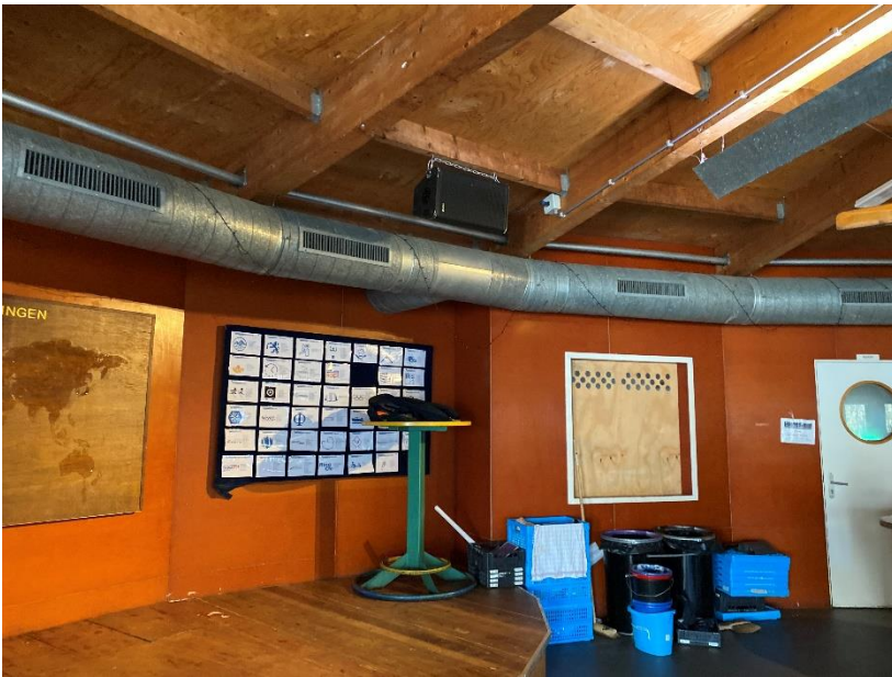
Figure 49 Mechanical supply duct in bar attic [own picture]
