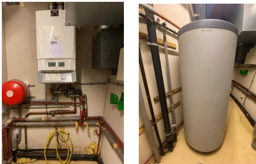
Figure 43 Gas boiler and hot water tank. [own pictures]
