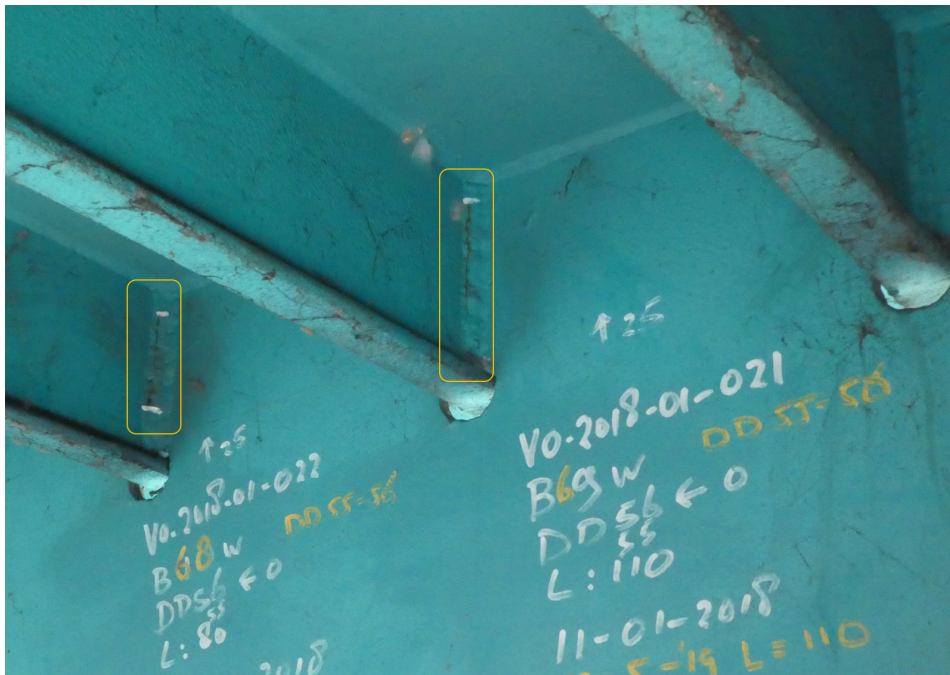
Figure 3.4: Fatigue Cracks Number 21 and 22 between the stiffeners and the transverse beam
