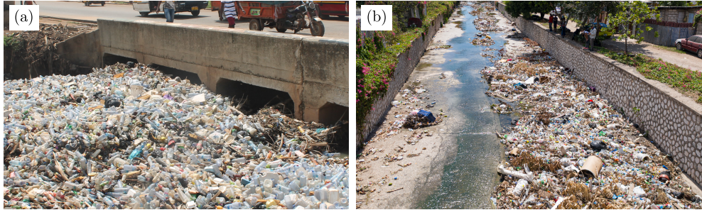
Figure 1.2: Accumulation of macroplastic debris at hydraulic structures: (a) waste accumulation at a culvert in Ghana (photo: Delft Global Initiative), and (b) waste accumulation in an urban drainage system in Jamaica (photo: The Ocean Cleanup).
