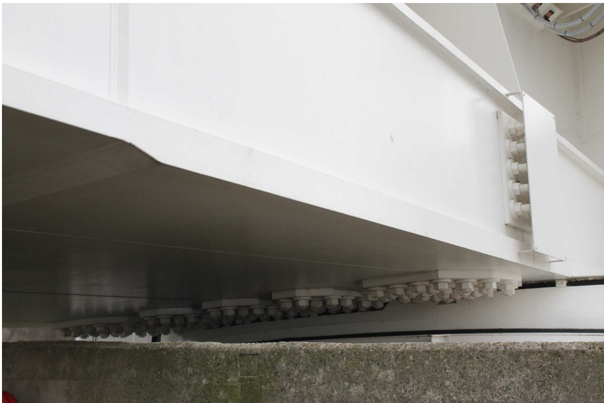
Figure 10 – Detail image of resin-injected preloaded bolts in the Maeslant Storm Surge Barrier [75]
