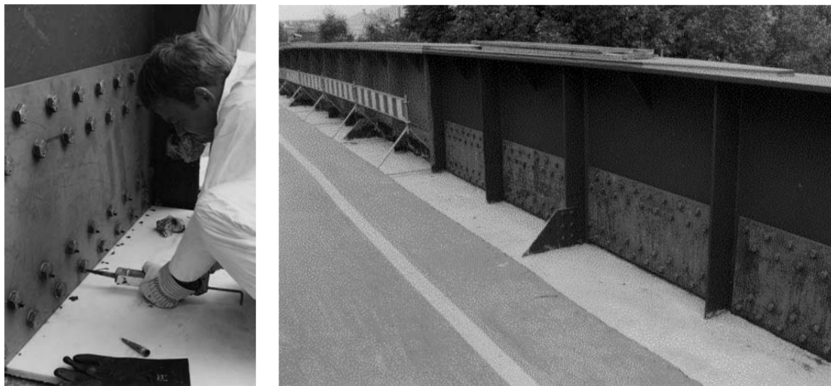
Figure 8 - Injection bolts in the Schlossbrücke Oranienburg (Germany). Left: injection process, Right: general overview of the final result [60]
