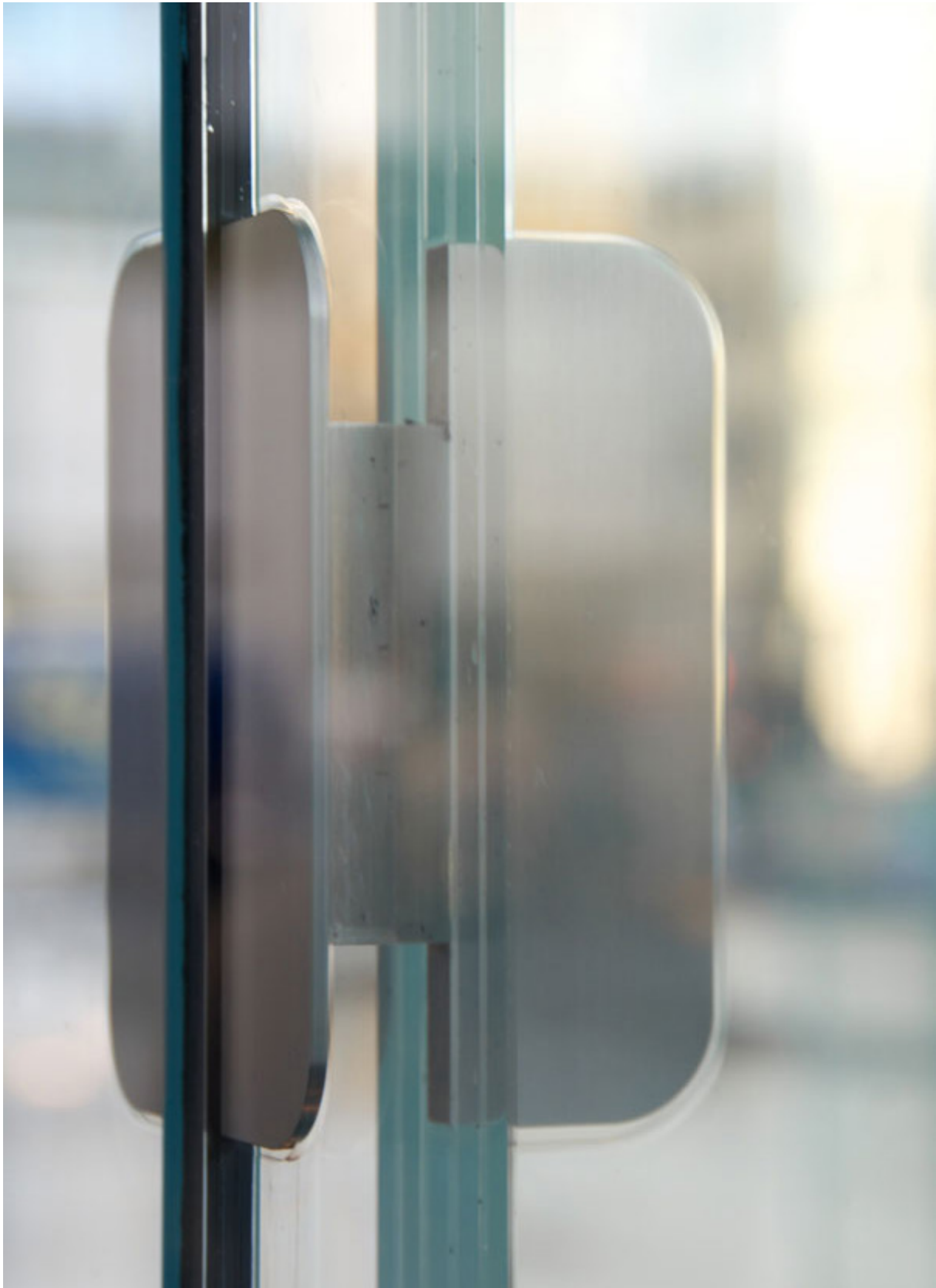
Figure 40: Embedded connections between column and facade panels in Apple Store in Fifth Avenue, NY. Source: https://www.eocengineers.com/en/projects/apple-fifth-avenue-mark-ii-100
