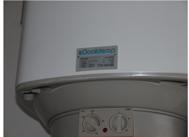
Figure 4-41: Domestic hot water boiler in kitchen
