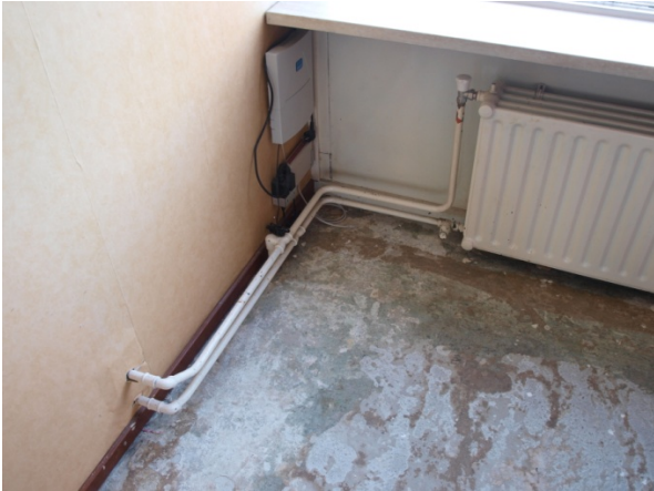
Figure 4-40: Radiator in living room
