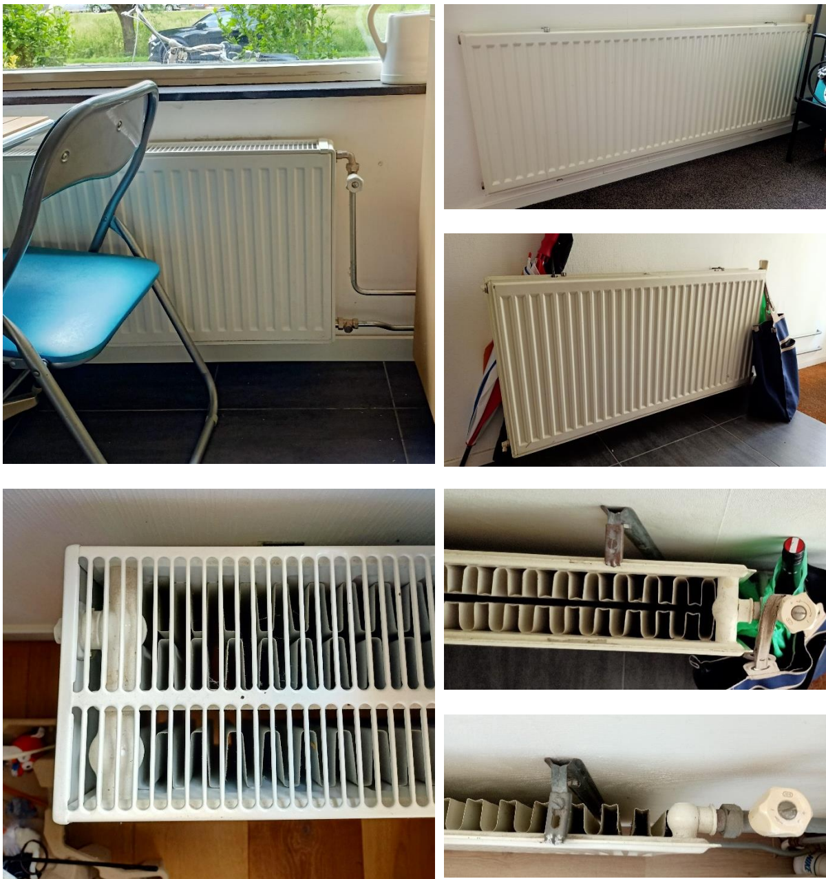
Figure 16.3: Overview of radiators
