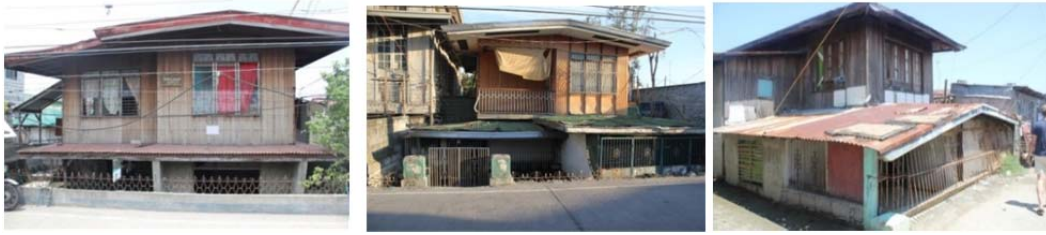
Figure 4.4: groundsubsidence in Hagonoy
