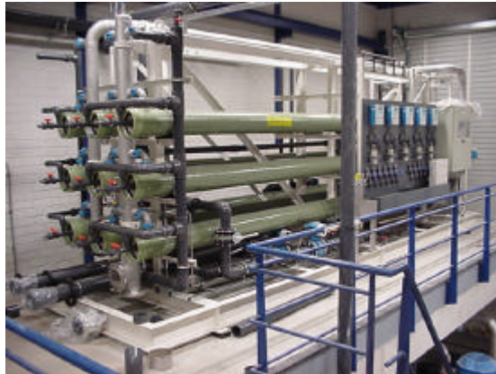
Figure 5. The Rodenmors nanofiltration plant (Vitens).
