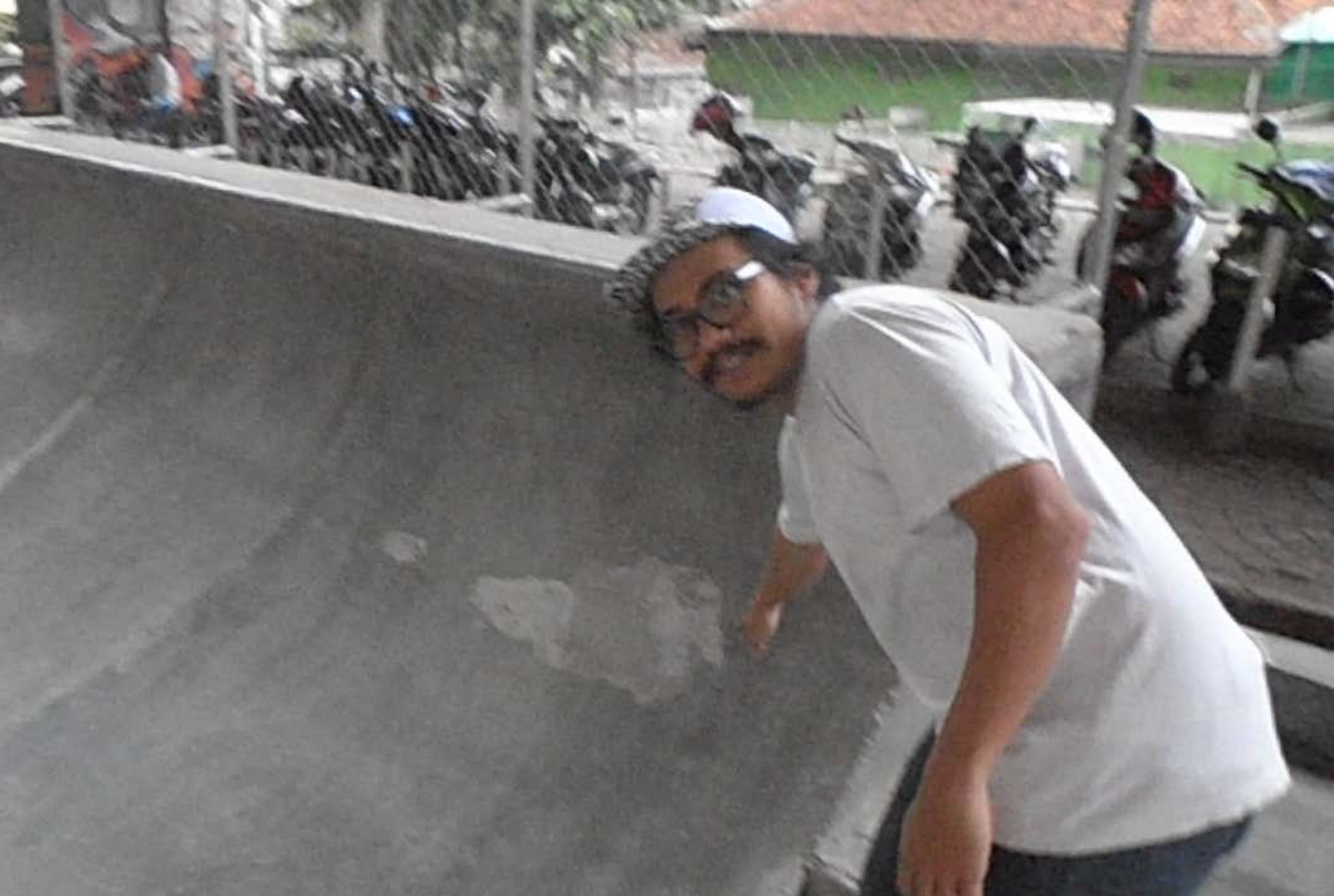
PROBLEM STATEMENT / Pasupati skatepark // Poor quality construction
