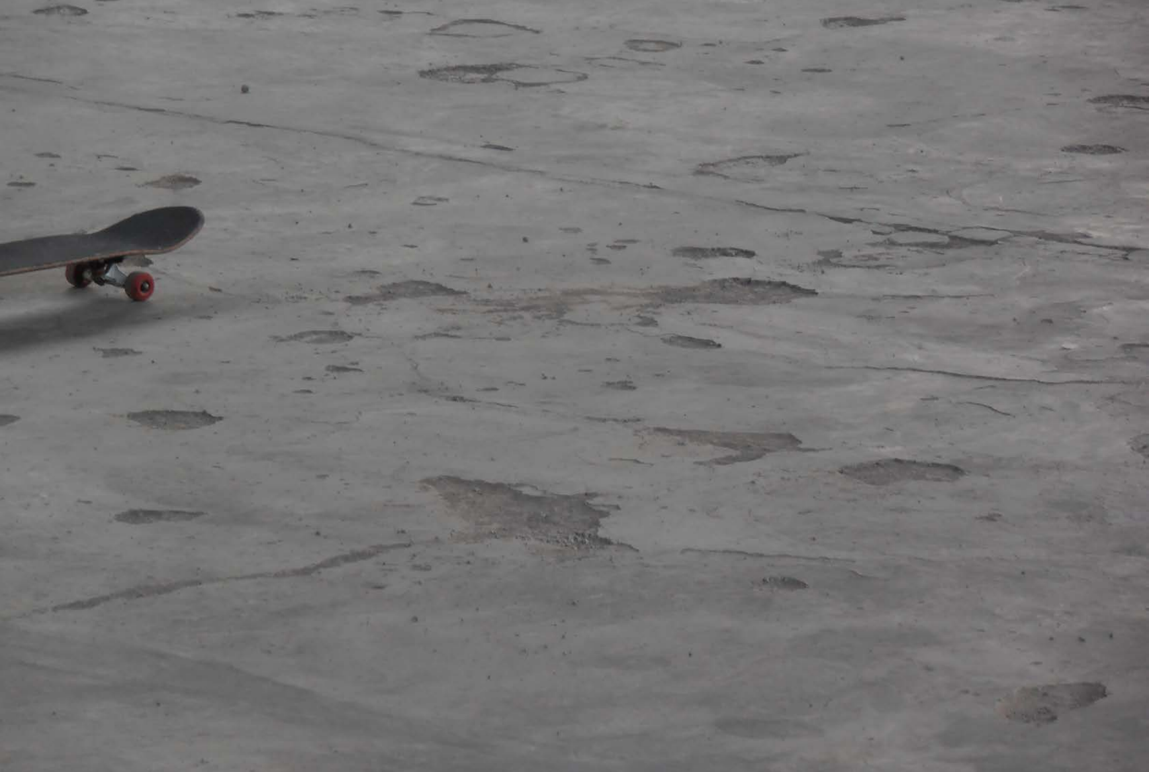
PROBLEM STATEMENT / Pasupati skatepark // Poor quality construction
