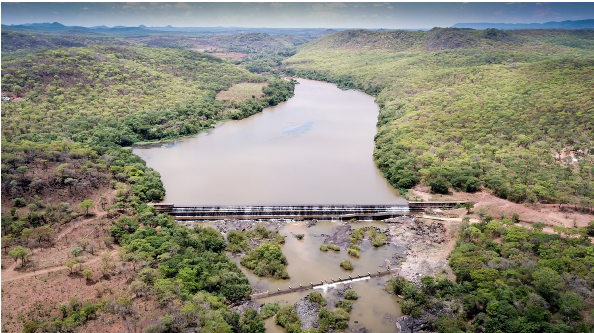
Figure 17: The Manyame Balancing Weir located in the MMSC
