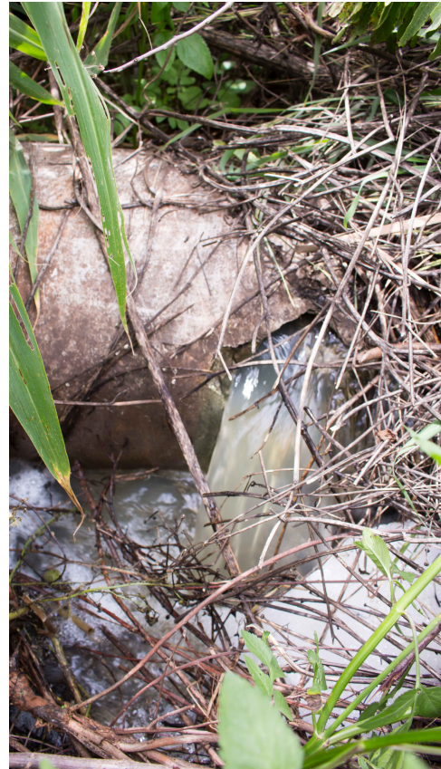
Figure 46: Leaking sewage effluent pipe in Chinhoyi (sample location 2)
