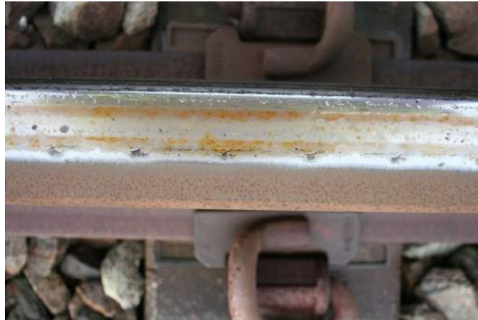
Figure 2: Example of RCF at a rail, which is visible as small cracks at the rail surface.
