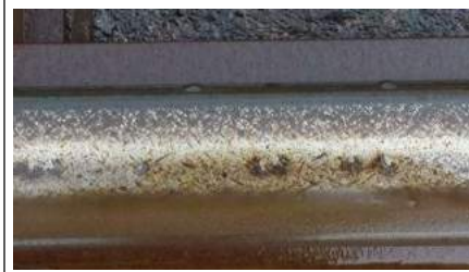
Figure 67: Close-up of the damages at Zoetermeer, we see the cracks here at the rail head.
