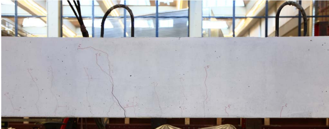
Fig. 5.76.1. Crack pattern after failure front side
