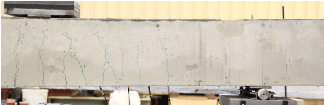
Fig. 5.22.2. Crack pattern after failure south side
