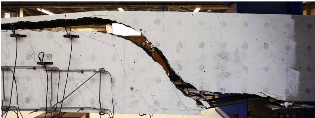
Fig. 5.106.2. Crack pattern after failure and part of LVDT layout at west side of beam
