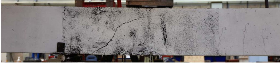
Fig. 5.75.1. Crack pattern after failure front side
