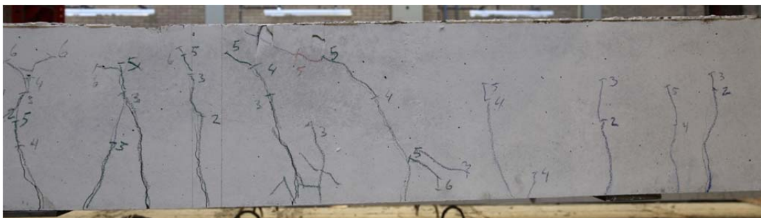
Fig. 5.36.2. Crack pattern after failure south side. (Picture taken after test A602A3.)
