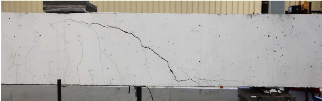
Fig. 5.46.2. Crack pattern after failure south side
