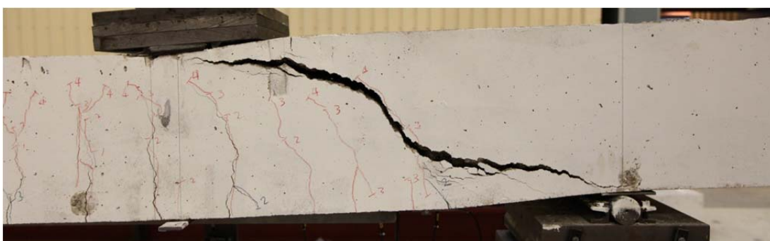
Fig. 5.68.2. Crack pattern after failure south side
