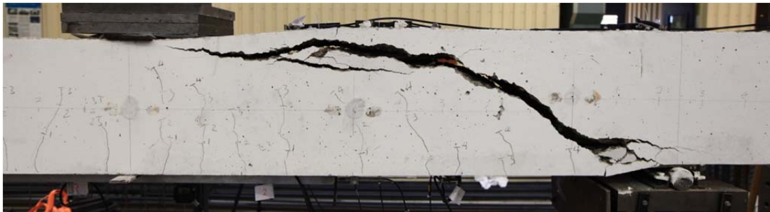
Fig. 5.57.2. Crack pattern after failure south side
