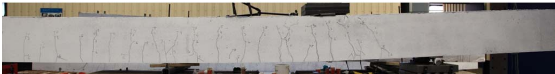
Fig. 5.35.2. Crack pattern after failure south side
