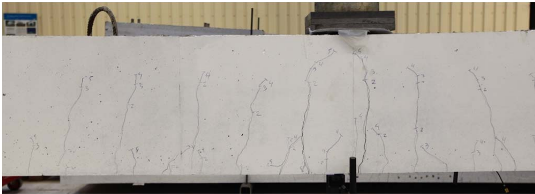
Fig. 5.47.2. Crack pattern after failure south side
