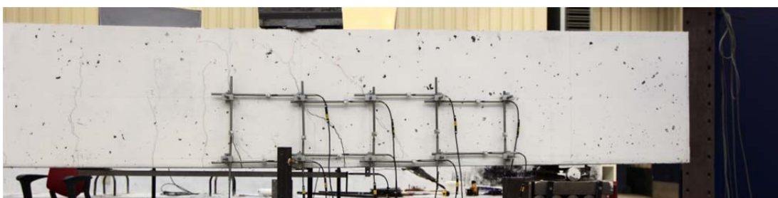
Fig. 5.81.2. Crack pattern after failure back side
