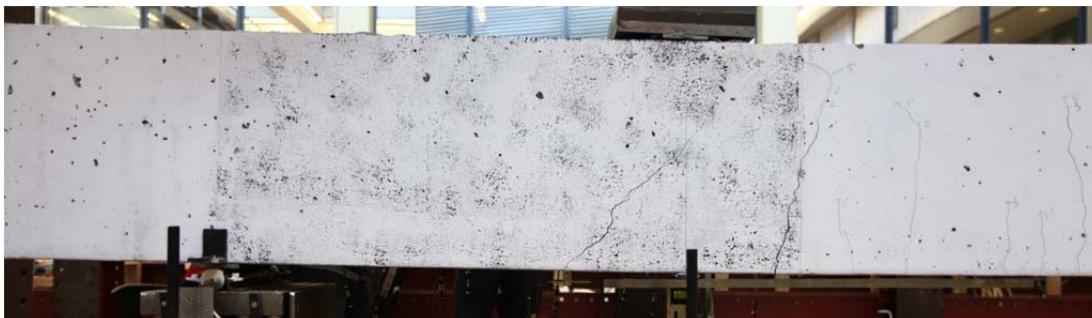
Fig. 5.81.1. Crack pattern after failure front side
