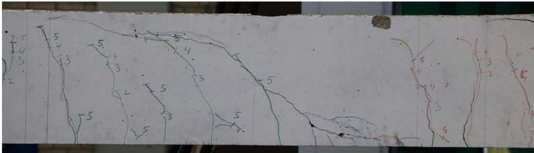
Fig. 5.27.2. Crack pattern after failure south side
