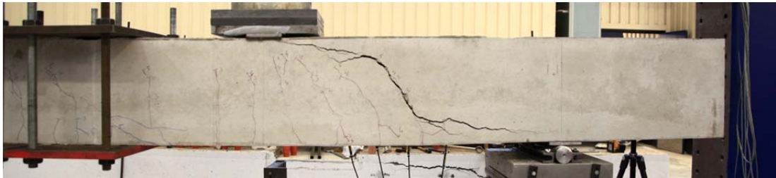
Fig. 5.25.2. Crack pattern after failure south side
