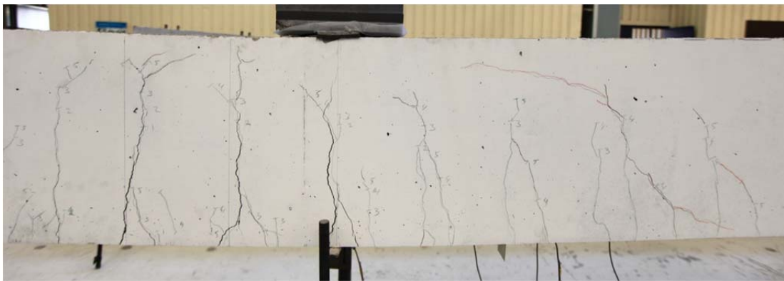
Fig. 5.42.2. Crack pattern after failure south side
