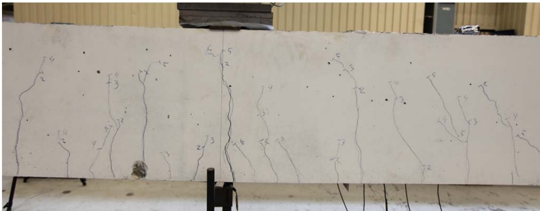
Fig. 5.43.2. Crack pattern after failure south side
