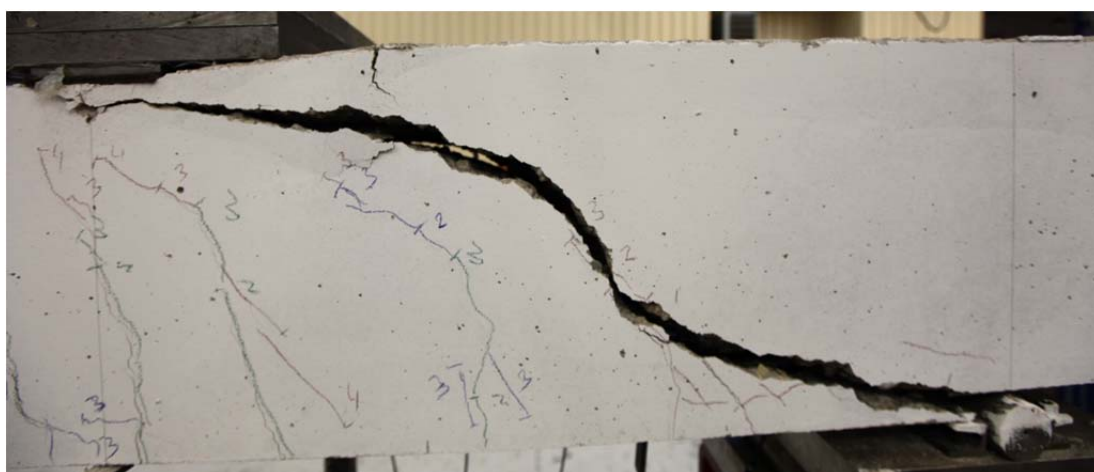
Fig. 5.64.2. Crack pattern after failure south side
