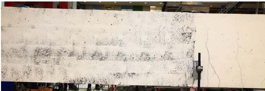
Fig. 5.92.1. Crack pattern after failure east side
