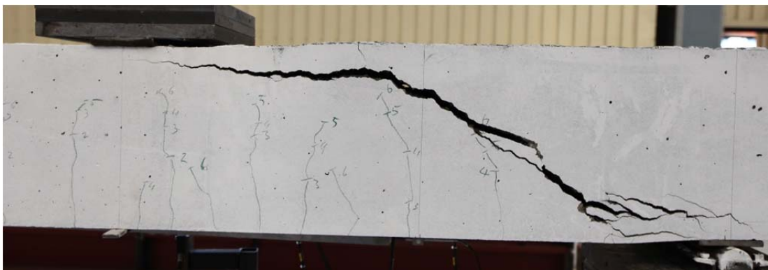
Fig. 5.8.2. Crack pattern after failure south side
