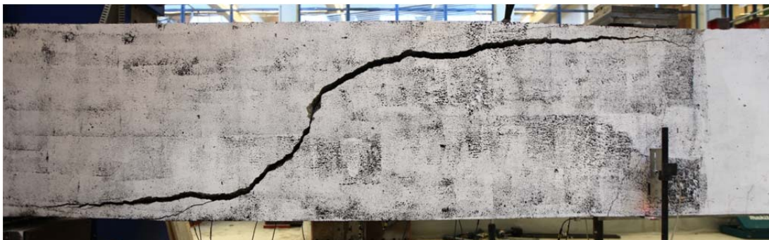
Fig. 5.91.1. Crack pattern after failure north side
