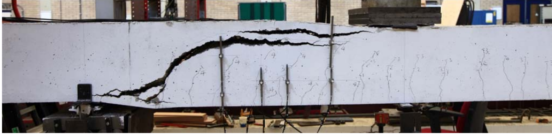
Fig. 5.57.1. Crack pattern after failure north side
