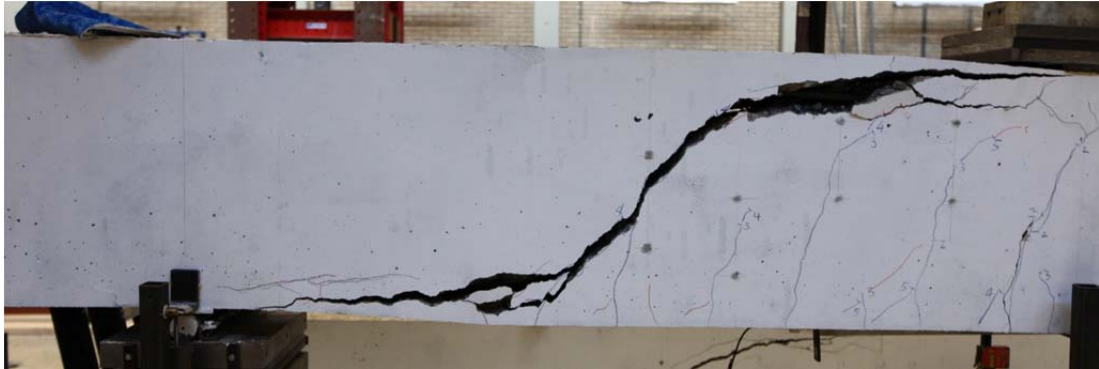
Fig. 5.52.1. Crack pattern after failure north side
