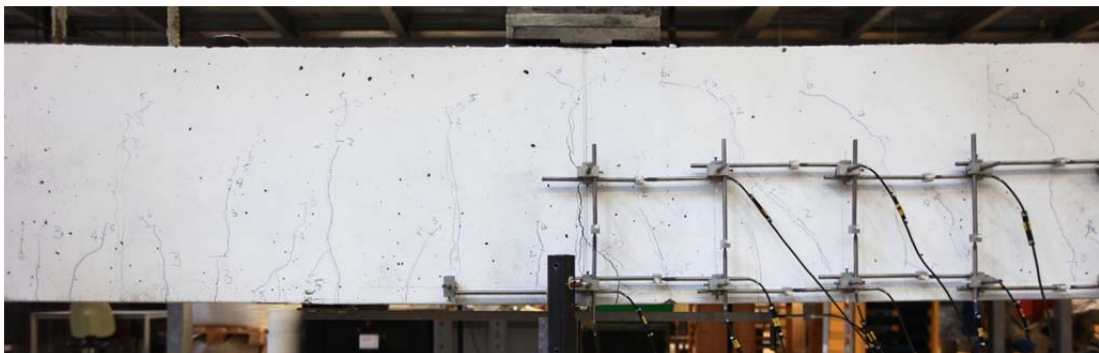
Fig. 5.97.2. Crack pattern after failure south side
