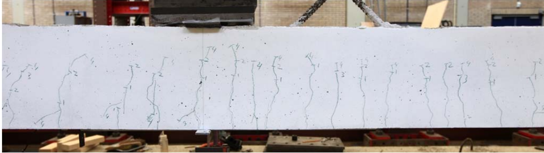
Fig. 5.58.1. Crack pattern after failure north side
