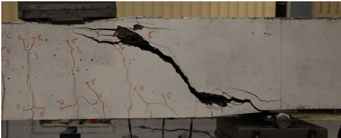
Fig. 5.33.2. Crack pattern after failure south side
