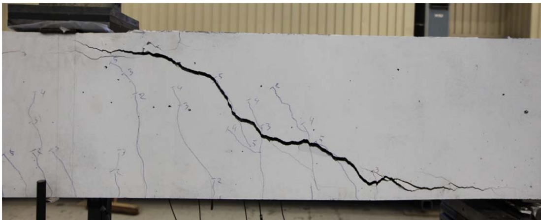
Fig. 5.44.2. Crack pattern after failure south side
