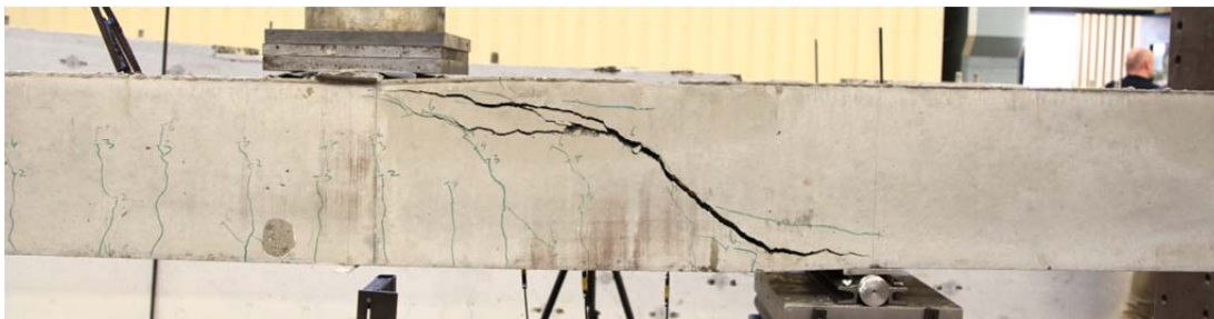
Fig. 5.15.2. Crack pattern after failure south side
