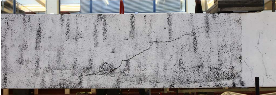
Fig. 5.95.1. Crack pattern after failure north side
