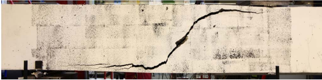
Fig. 5.99.1. Crack pattern after failure east side
