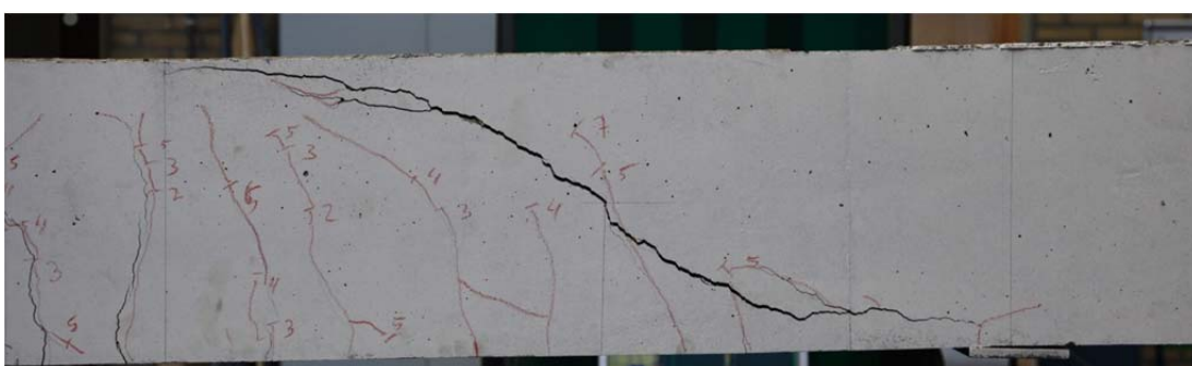
Fig. 5.28.2. Crack pattern after failure south side
