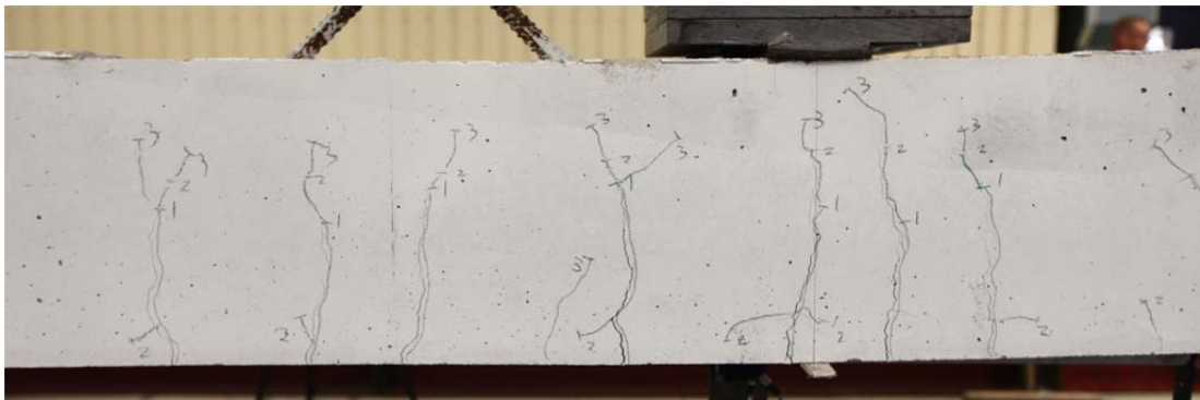
Fig. 5.62.2. Crack pattern after failure south side
