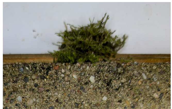
Fig. 9. The mosses that lost adhesion to the concrete surface still appeared healthy in most cases.
