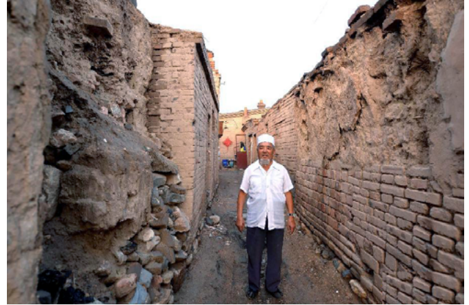
Fig. 5-3-1: Baotou Beiliang Hui Nationality historical area (200 years old) _(Residential buildings are seriously damaged by the rainstorm) Source: http://news.xinhuanet.com/photo/2013-09/02/c_125301035_3.htm
