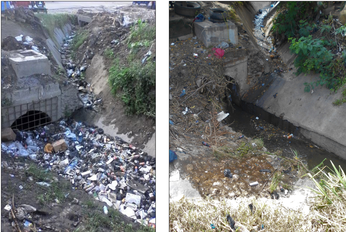
Figure 3.10: Drain at Africa Sana, in the crossroad Shekilango road/Mabatini road. Left image: 28 September 2015, http://ramanihuria.org/mapping-drainage-in-dar-es-salaam/ . Right image: 6 March 2019, photo by the author.
