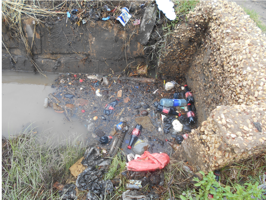
Figure 5.15: Culvert blocked by plastics the morning after the simulated event.
