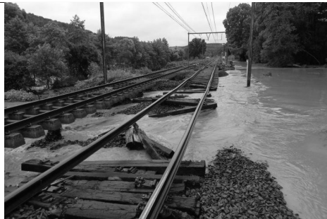
Figure 2.1.13. Photo of flood damage to railway in Maastricht Source: Google Images (1993)
