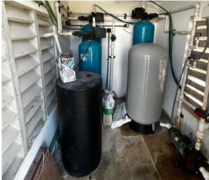
Figure 3.9: The water softener of Well 3 where freshwater is extracted.
