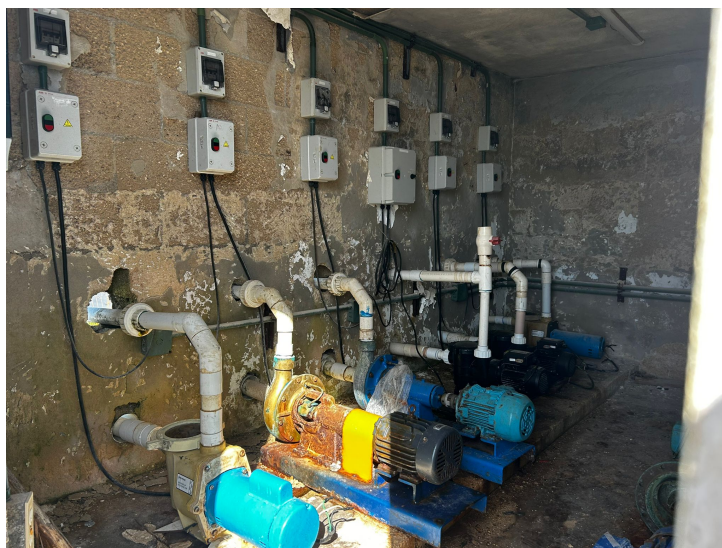
Figure 3.10: Pumps of Well 1 that extract saltwater.
