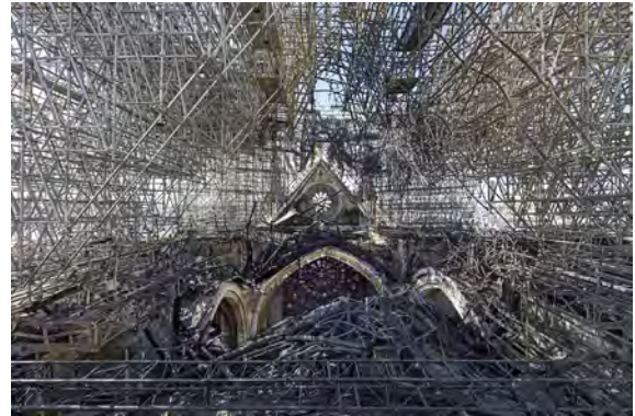
Figure 7 Unstable, partly melted aluminum scaffolding structure (New York Times, 2020).
