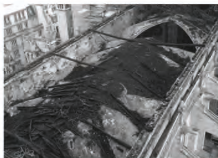
burned down timber debris on top of vaults
