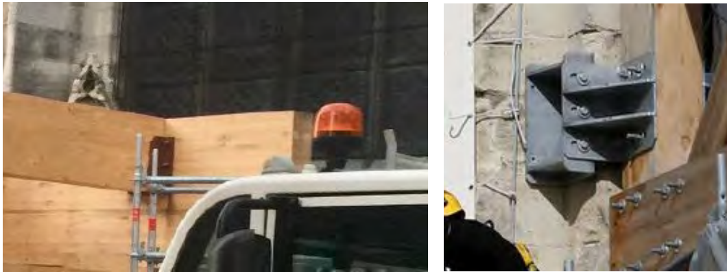
Figure 54 Joint types used by authorities: left: Joist hangers used to connect members of cassettes. right: Steel clamping connections located underneath flying buttresses.
