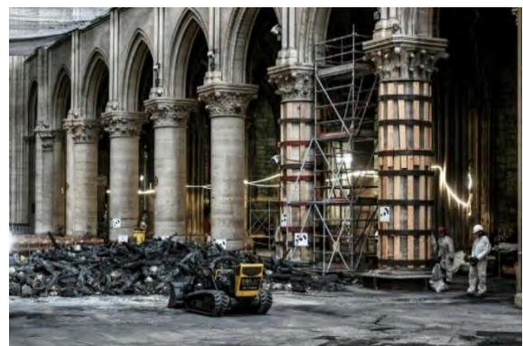
Figure 9 Burned oak beams fell through the vaults and damaged the interior (New York Times, 2020).
