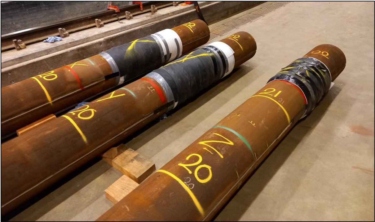
Figure 4.8: Protecting the loose fibre optic cables at the pile heads using foam and rubber mats
