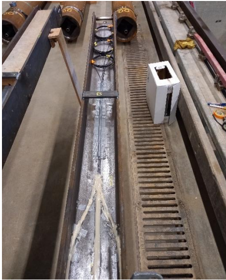
Figure E.2: Head of the H-beam reinforcing of an SI pile. The reinforcing of the SI piles had a free length of 1-2m, part of which was cut off after installation. As a result, the highest glued point of the fibre optic cables was set conservatively.
