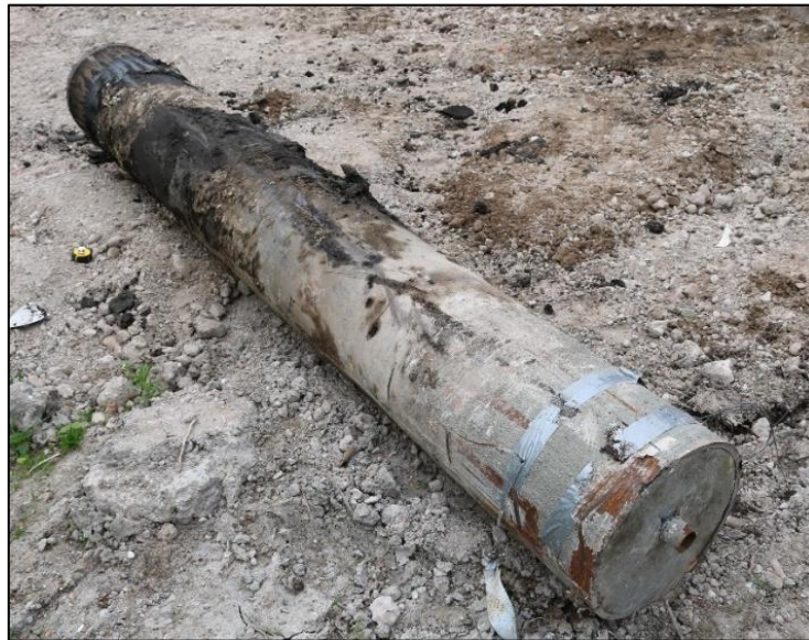
Figure 4.12: Head of pile T1 after extraction. No clear evidence of grout was present at the head of any of the SIC piles
