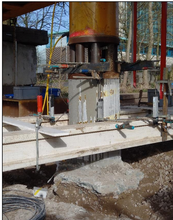
Figure 5.43: Pile F2 prior to testing. Note the grout shell at the base of the pile cap
