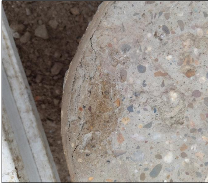
Figure 5.14: Cracking in the head of pile F1 on the surface of the pile head, at its north-western side
