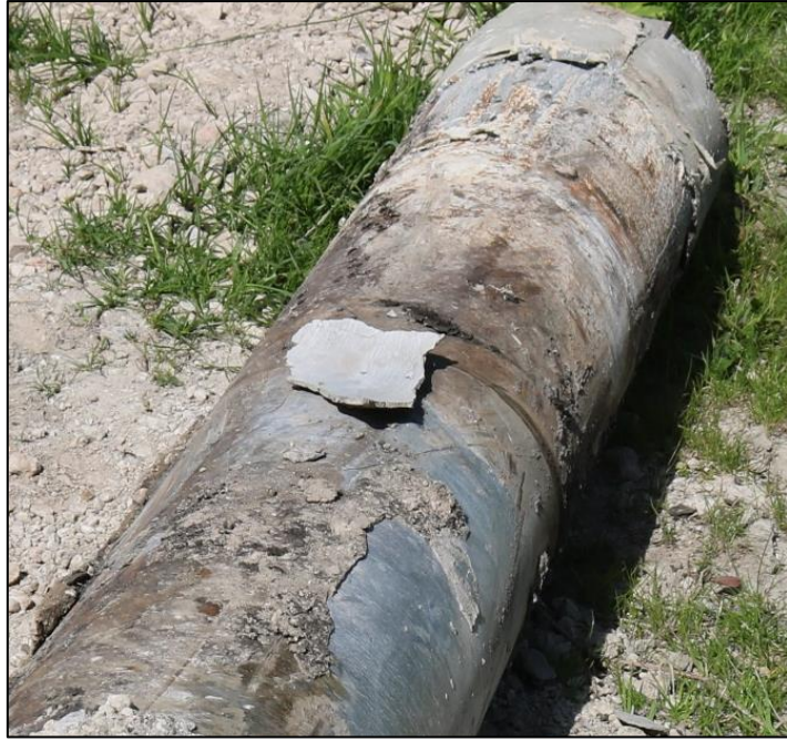
Figure 4.14: Close-up of the head of pile F3, with one of the broken pieces placed on top of the pile
