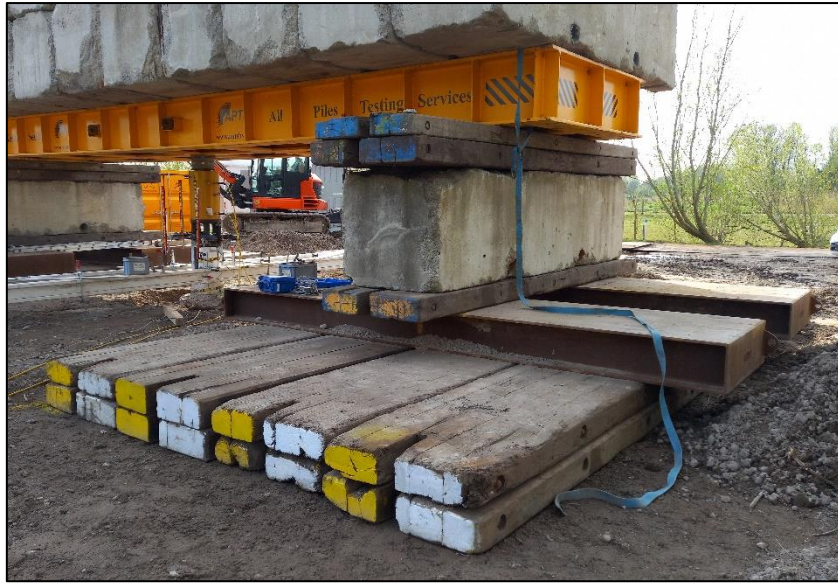
Figure E.5: Footing configuration for each test. The number of dragline mats between the concrete block and the frame was changed from test to test to ensure enough height above surface level was provided
