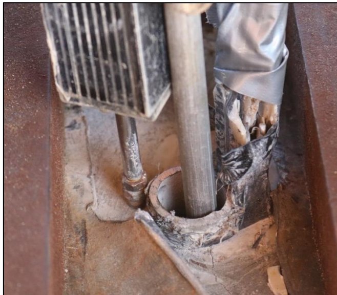
Figure 5.72: Sharp bending in the FO cable of pile F3, leading to loss in light intensity and reduction in measurement quality
