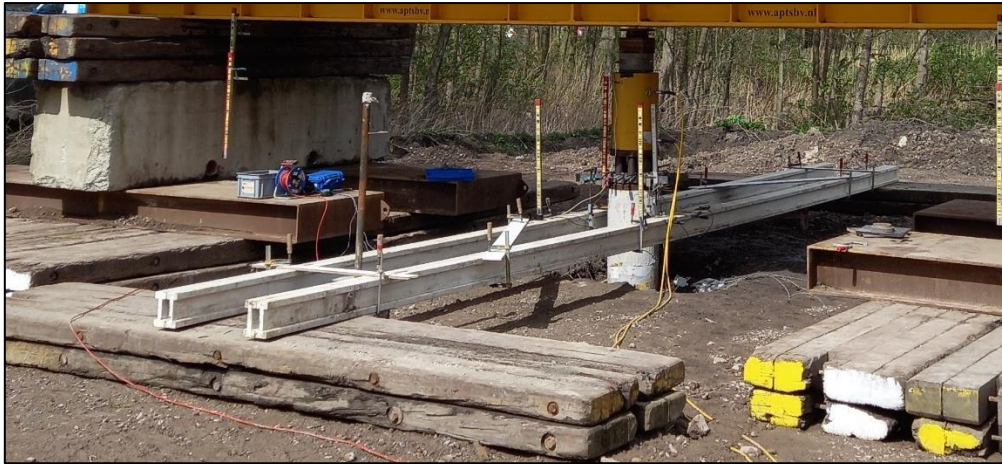
Figure 7.5: Reference frame, resting on dragline mats, each 5.5m away from the pile
