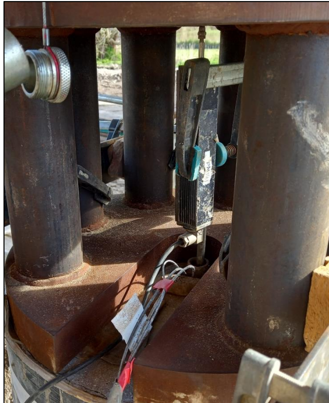
Figure 5.44: Placement of the telltale PM for pile F2. The platen is touching the top side of the transition piece
