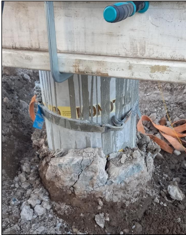
Figure 5.71: Cracked grout at pile head
