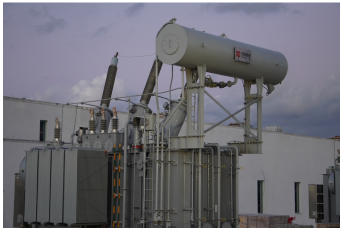
Figure 55. High to medium voltage transformation
