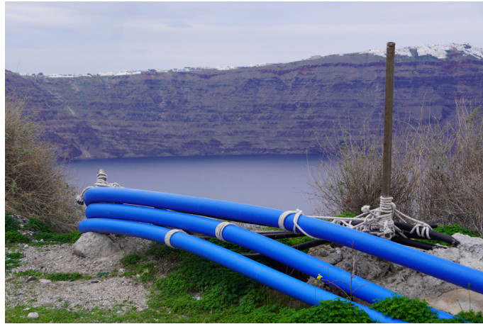
Figure 59. Pipes over the cliff
