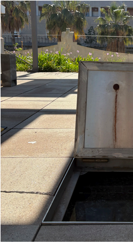
Water underneath the e
