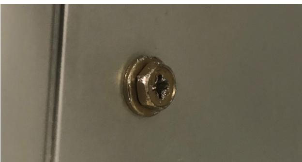
Fig 3.5. Worn out bolts
