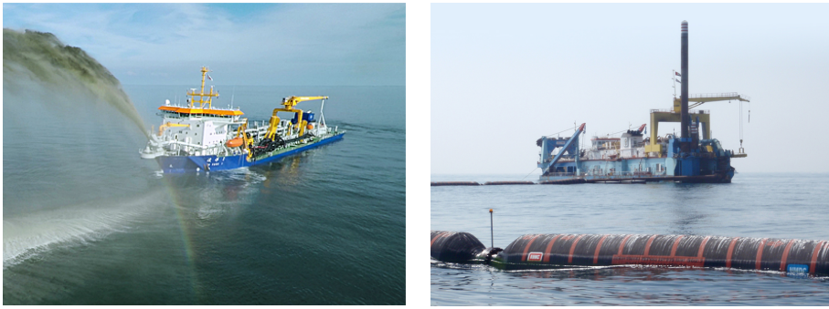
(a) Rain-bowing by a Trailing Suction Hopper Dredger (source: Royal IHC). (b) A Cutter Suction Dredger discharging on a floating pipeline (source: Royal IHC).
