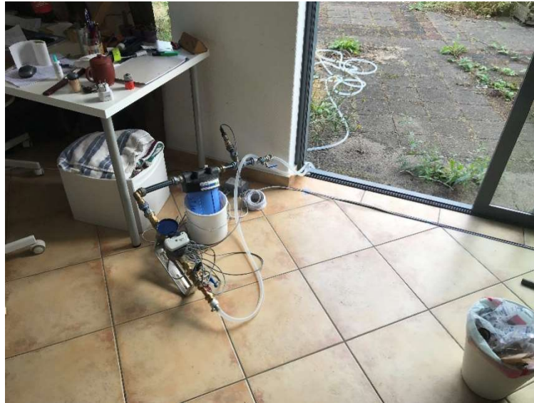
Figure 3-15 Smart Water Meter in Delftgauw.
