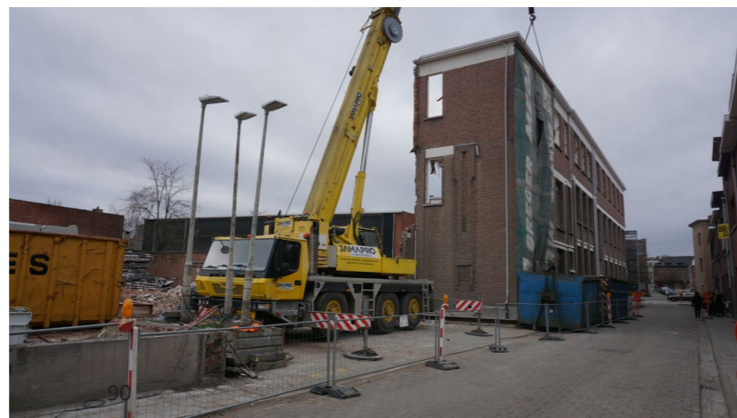
Entering the demolition site. Where the big truck and street posts are now standing, there used to be part of the building that has been taken down already.
